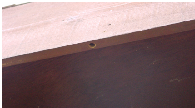
Figure 2. Carpenter bee entrance hole in fascia.
