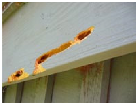
Figure 4. Carpenter bee gallery exposed in wood.
