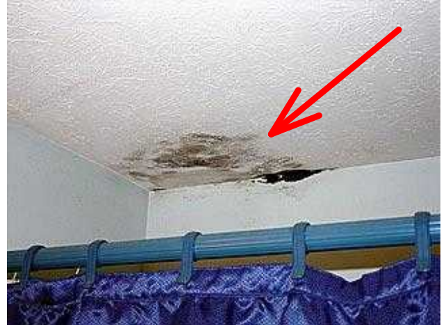
Possible visible mold and water leak
