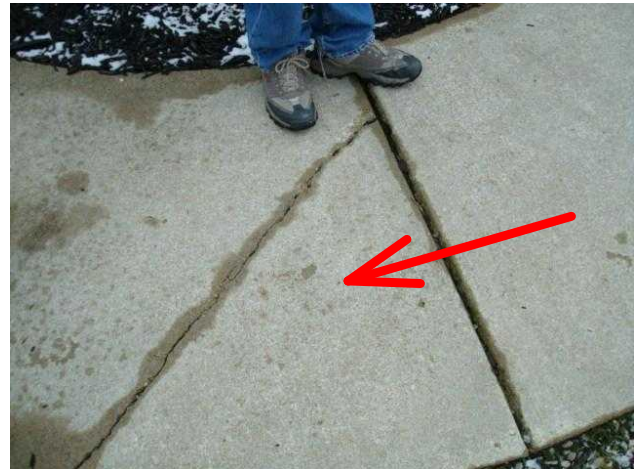
Settlement in the sidewalk
