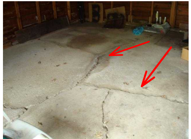
Garage floor cracked with displacement
