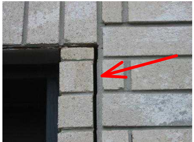
Separation of brick at window
