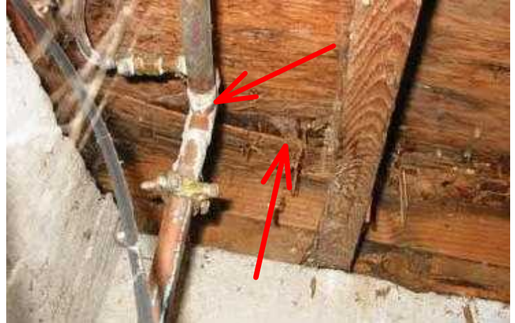
Wood rot and possible plumbing leak
