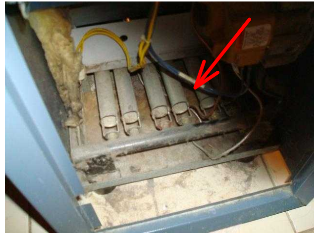
Boiler needs cleaned and serviced and heat exchanger checked for cracks.
