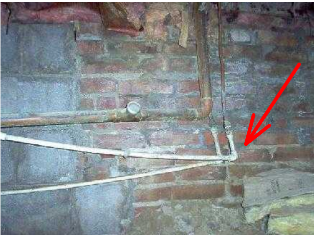
Pipes are not secure and leaking
