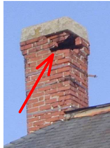
Bricks missing from chimney
