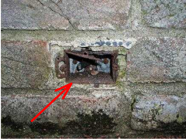
Outlet rusted out
