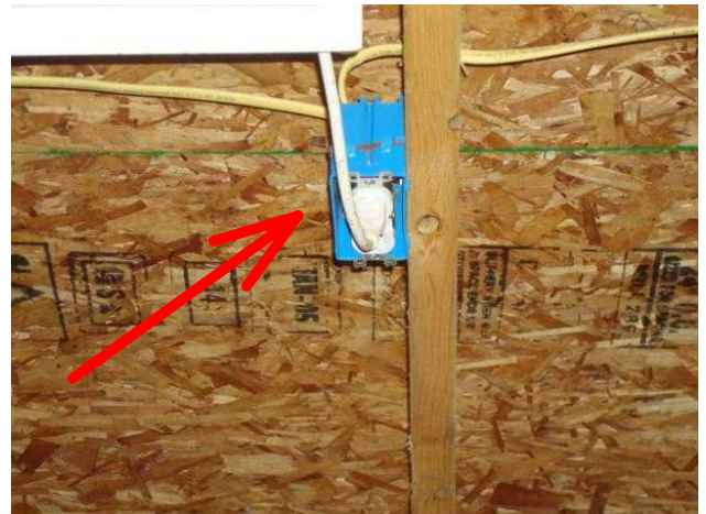
Outlet cover missing
