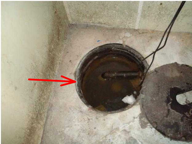
Sump pump inoperative
