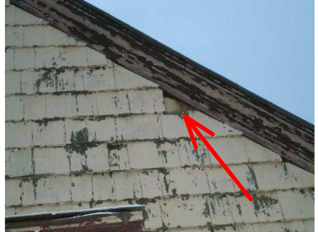
Missing siding and needs scraped and painted
