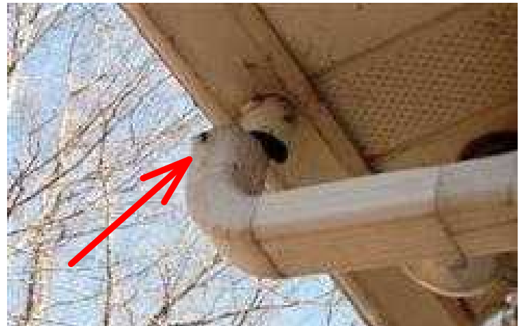
Down spout loose
