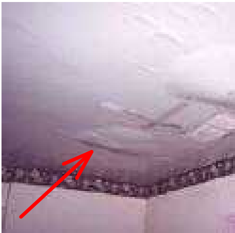
Water damage in living room ceiling
