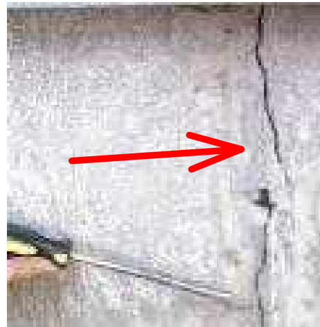
Foundation crack with displacement
